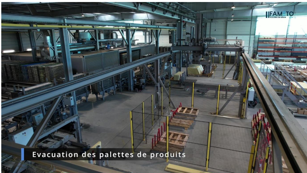
11. 11. Product output conveyor with turntable for bypass and waste output.
